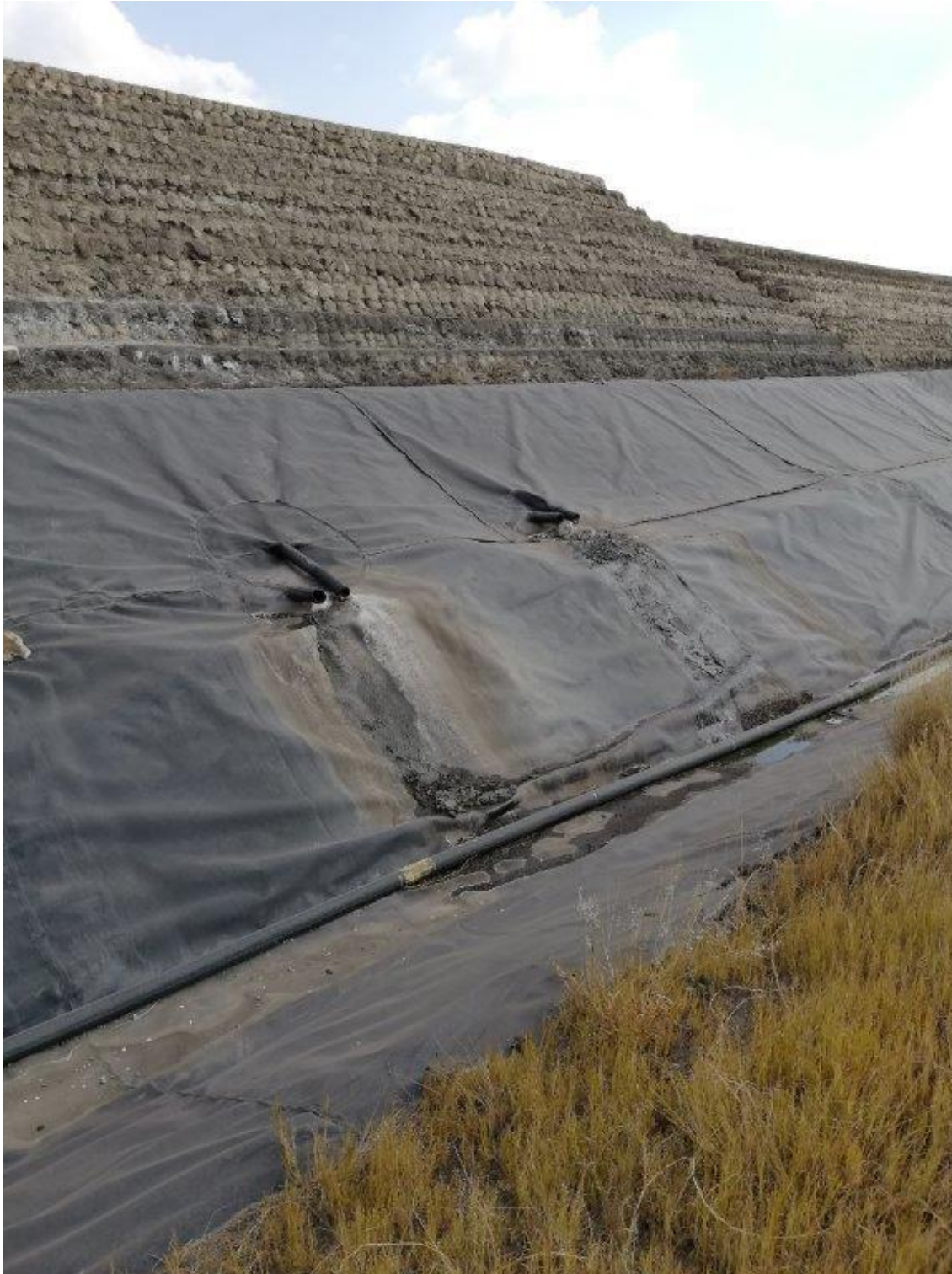
Figure 4: Seeping drainage pipes
