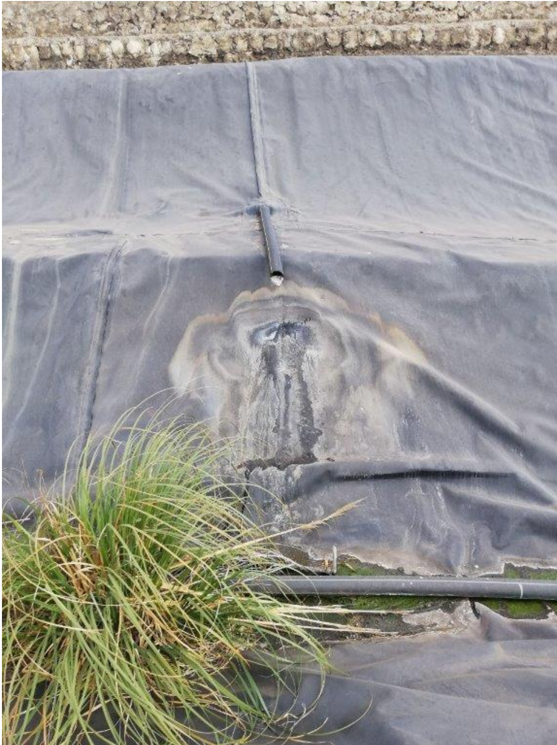
Figure 5: Seeping drainage pipe
