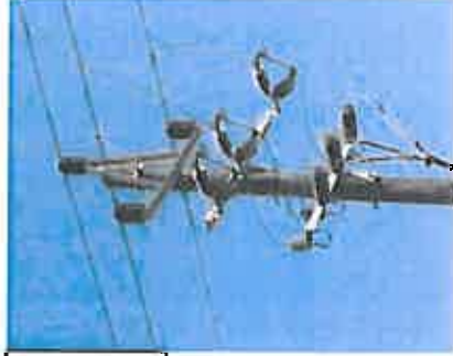
Figure 11: Typical 22KV single Power line
