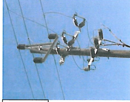
Figure 11: Typical 22KV single Power line
