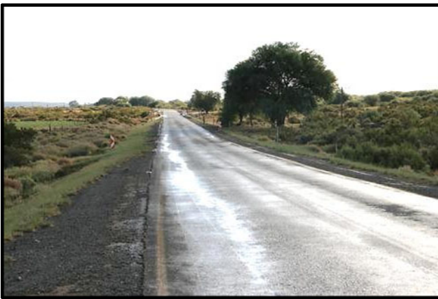
Figure 23. East side of Bridge 2 with disturbed road reserve colonised by weedy species. On the right hand side is a lay-by under the large thorn-tree.
