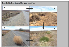
Photo 2 A. Team funded by Extended Public Works Programme clearing indigenous Karoo bushes from the roadside between east of Neuwoudville in the Nama Karoo on 11 March 2005. Note the low dense and brown colour of the vegetation. B. The Karoo bushes are not controlled but are cut at ground level. The roots of the plants at least reduce erosion of soil by wind and water. Piles of cut branches are stacked against the fence. C. Grasses and weeds (including the tall like Russian Timberrweed) obscure road verges near Williston that were cleared of indigenous shrubs about two months previously. Note that the bushes are larger and greener than the local Karoo bushes. They therefore obscure more of the road as well as attracting bees and other insects for green forage plants in this dry landscape. D. A dry Russian Timberrweed (Calceola Aul) that has broken the off the soil and is about to roll across the road. The bush although light in weight, measures 1 m in diameter and could easily cause a driver to swerve particularly if it bounces across a motorist's path at night. An old name for this plant is perdenbush.
