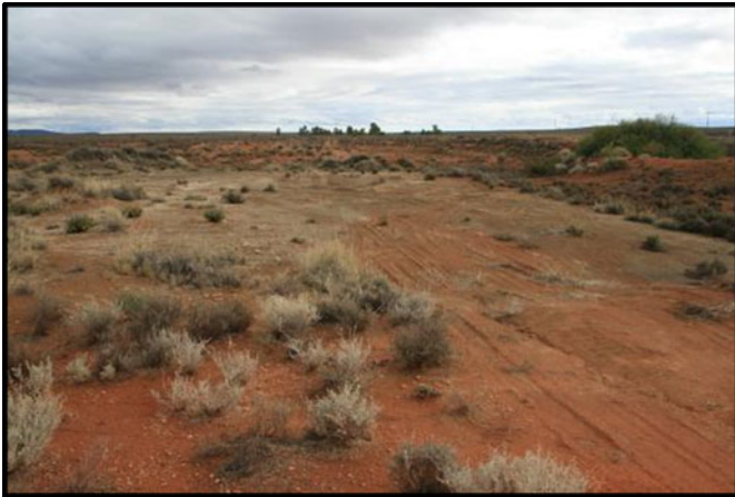
Figure 16. Borrow pit 5 which presently covers an extensive area would be extended southwards and also made deeper in places.
