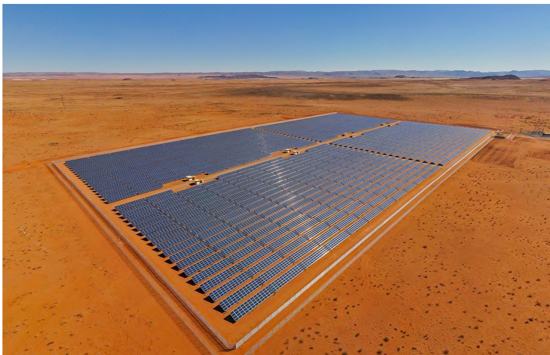
Figure 7: Konkoonsies Solar PV Plant on Portion 6 of Farm Konkoonsies 91 (Source: http://www.biothermenergy.com/blog/konkoonsies-solar-pv )
