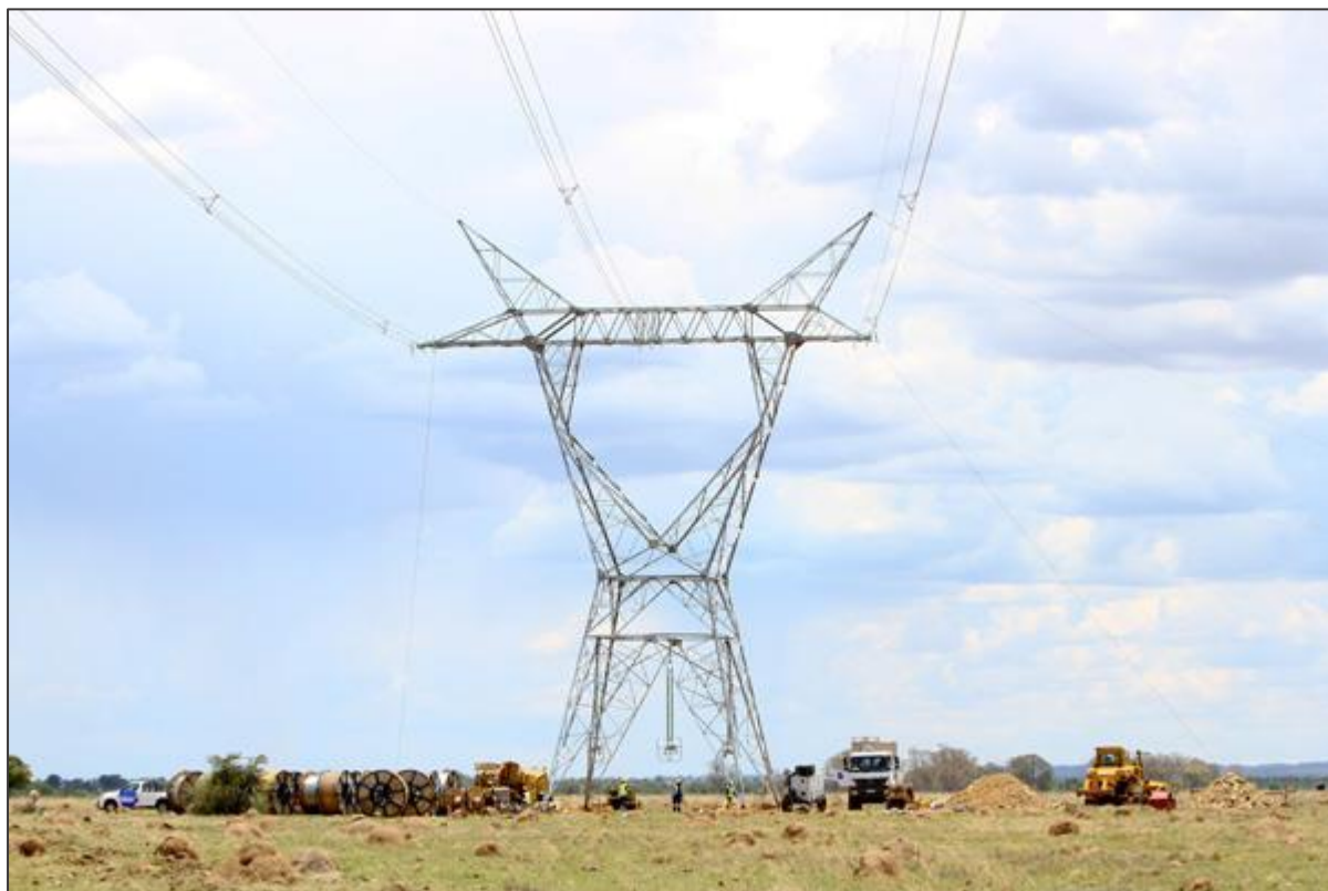
Figure 5.1: Stringing of power line infrastructure in South Africa.
