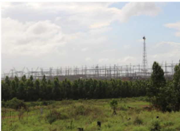
Plate 3 - Sub-station & Communication Tower
