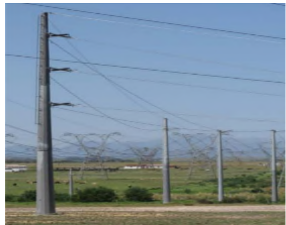
Plate 4 - 23-28m high, 132kV self-sustaining steel monopole tower.
