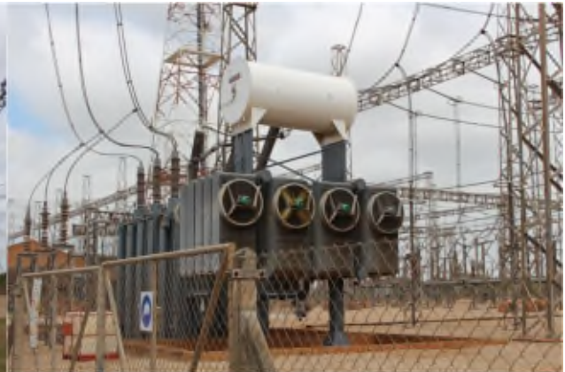
Plate 2 – Transformer with oil storage tank above.
