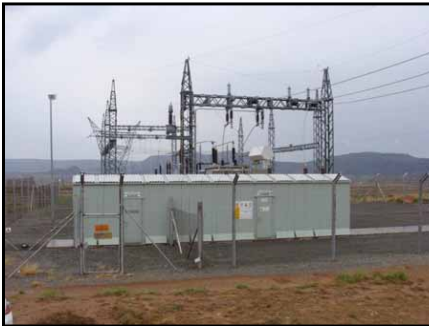
Photograph 1.1: Existing Ludlow substation located to the west of the site
