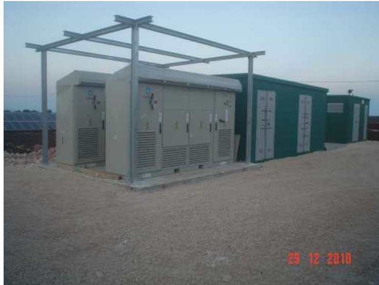
Figure 14 : Typical on-site substation
