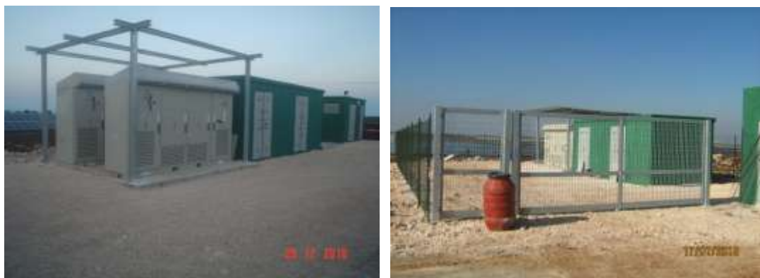
Figure 7: Typical on-site substation footprint
