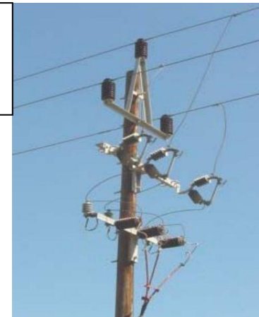
Figure 11: Typical 22KV single Power line
