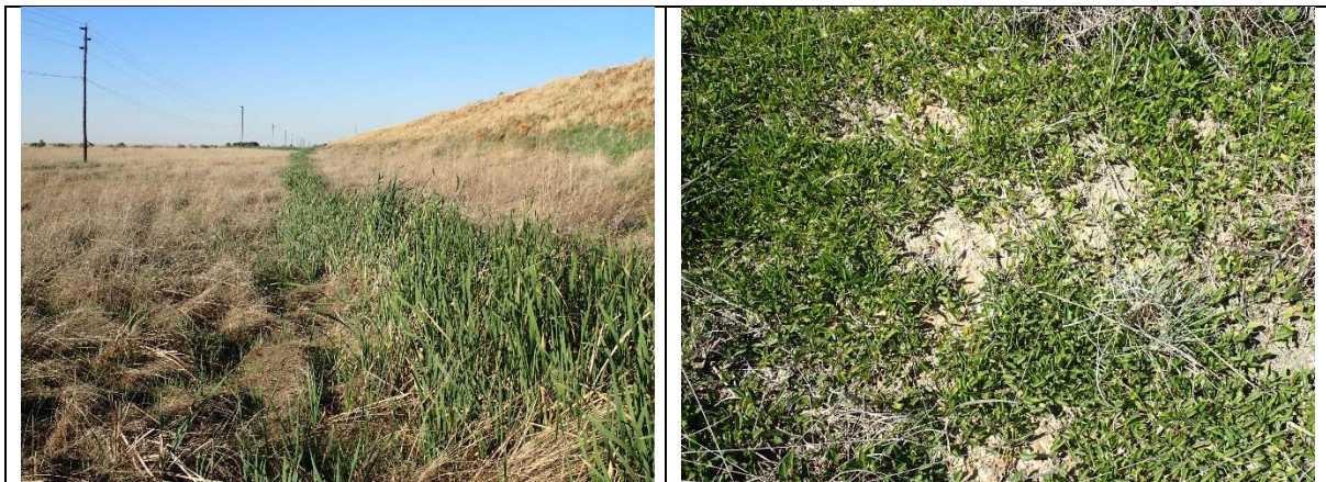
Figure 5: Toe seepage from the existing TSF into channelled valley bottom wetland 2 is visible along the edge of the footprint and the presence of a corresponding linear zone of Typha capensis , an obligate hydrophyte, in the northern section of the wetland (left); and evidence of tailing depositions within valley bottom wetland 2 downstream of the existing TSF in an area colonised by the hydrophyte Falkia oblonga (right).
