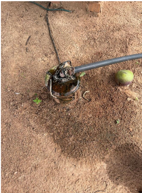
Photograph 6 – AC-06 (Private Borehole In use)
