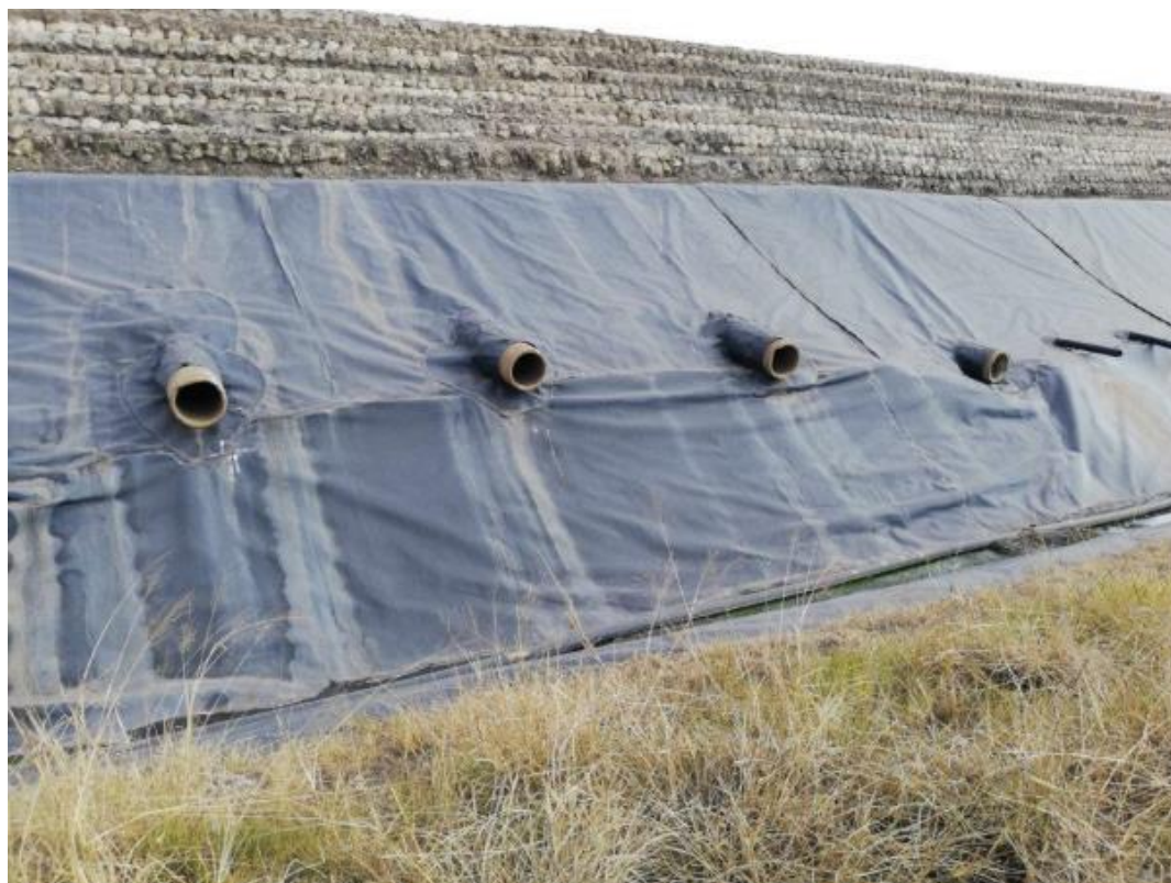
Figure 5: Penstock pipe outlets through starter wall
