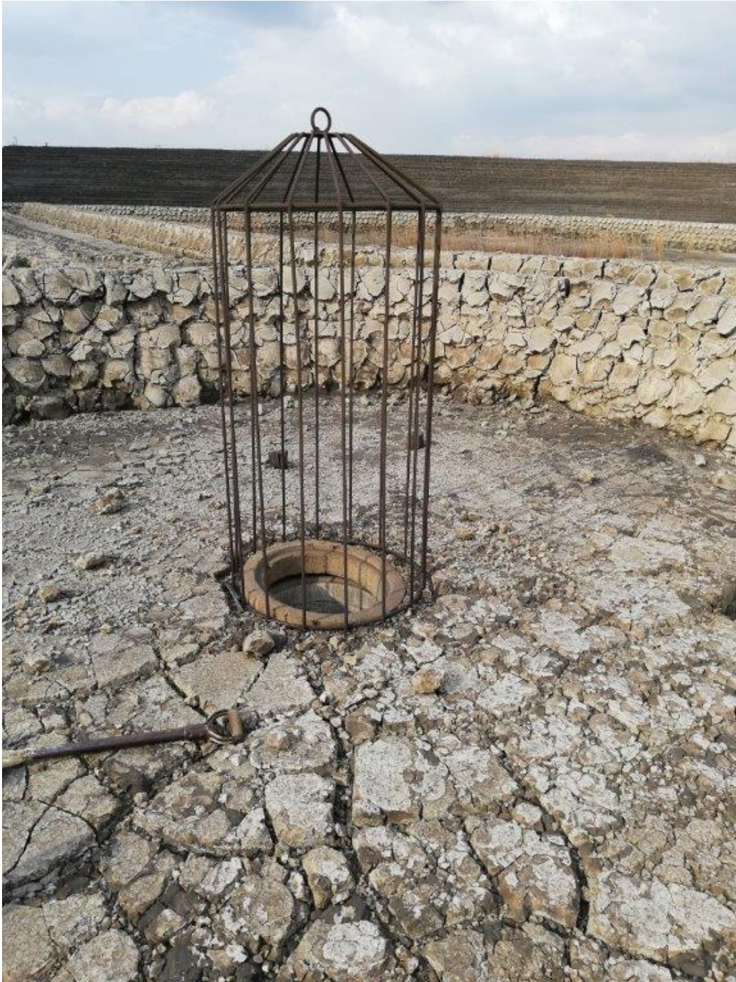
Figure 4: Penstock - North Dam
