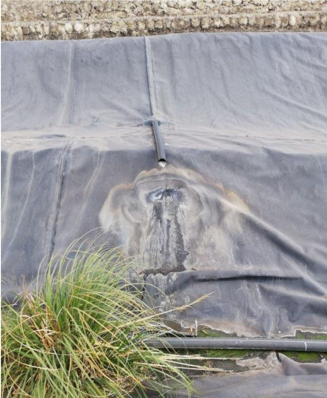
Figure 20: Minor seepage observed from Underdrainage pipes
