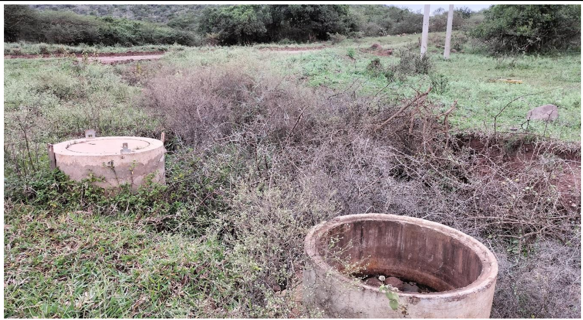
Civil infrastructure leading to head cut erosion and sedimentation (HGM 1)
