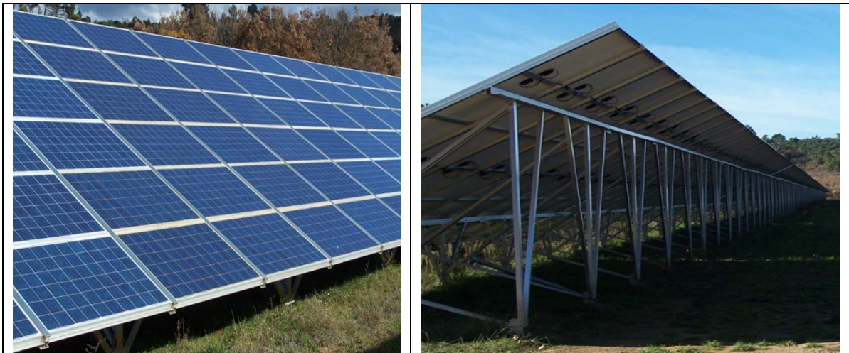
Figure 1.3: Illustration of photovoltaic panels
