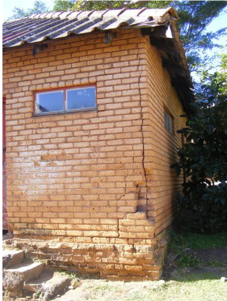
Fig 22: Showing structural cracks to corner of shed
