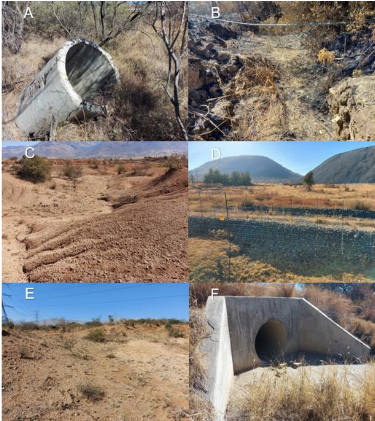
Figure 5-5 Aspects contributing to modifications to wetlands. A) Dilapidated infrastructure. B) Infrastructure crossings. C) Erosion. D) Roads and crossings. E) Infrastructure development. F) Stormwater networks
