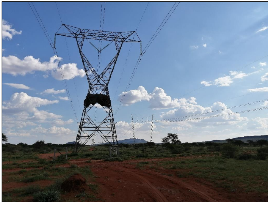
Figure 14: Existing 275kV line with a sociable weavers' nest.
