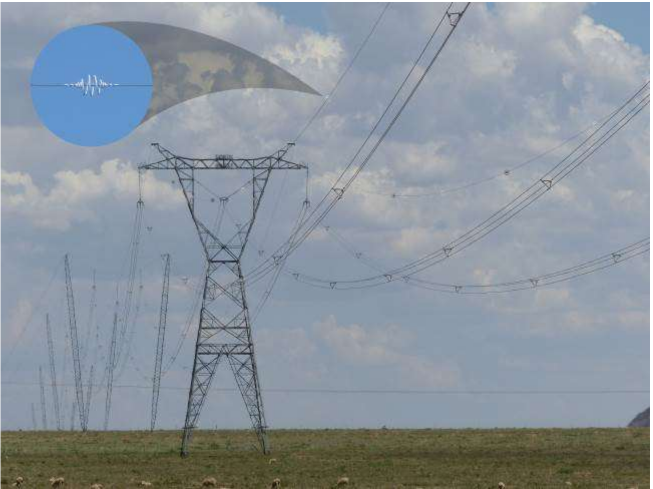
Figure 16: Example of bird flight diverters employed on the earth wires of a power line.
