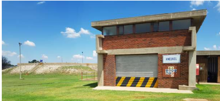
Figure 5: Kneukel Pump Station and Sump
