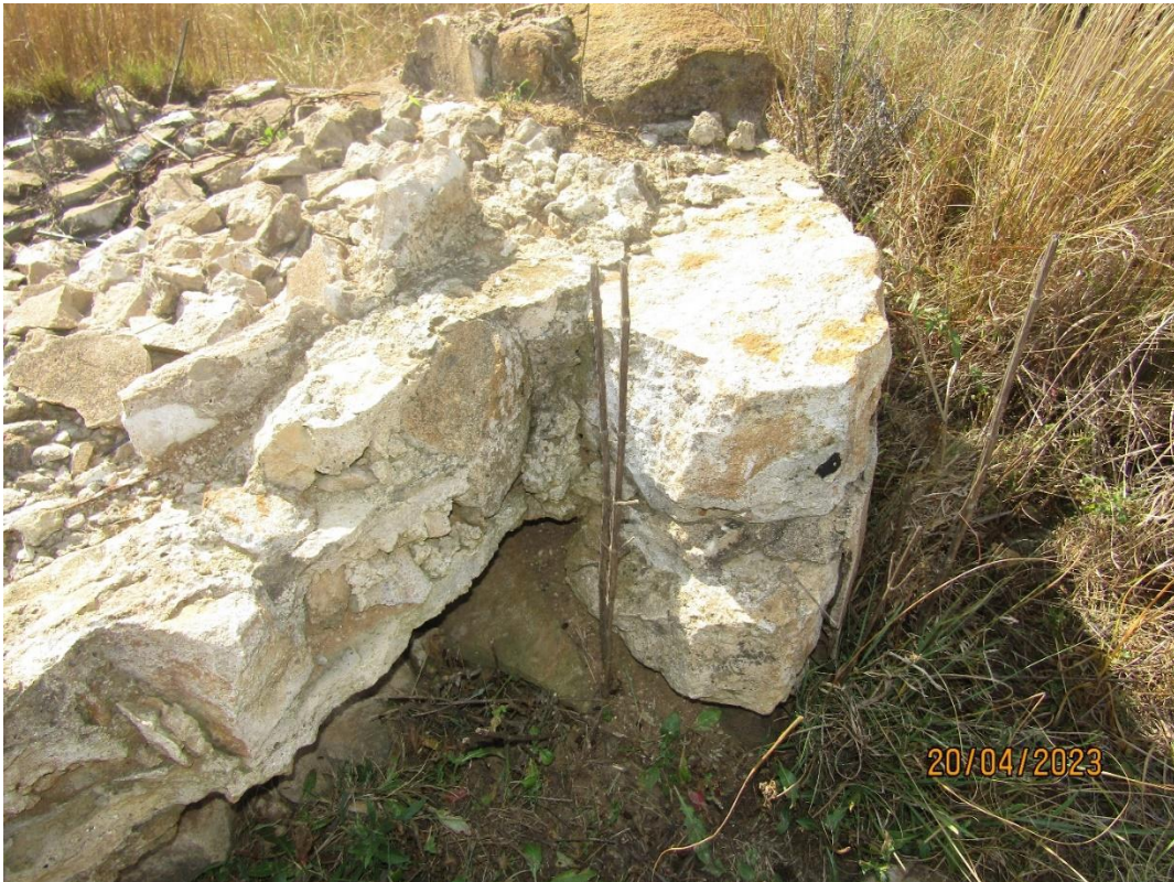
Figure 14: An old demolished water storage tank
