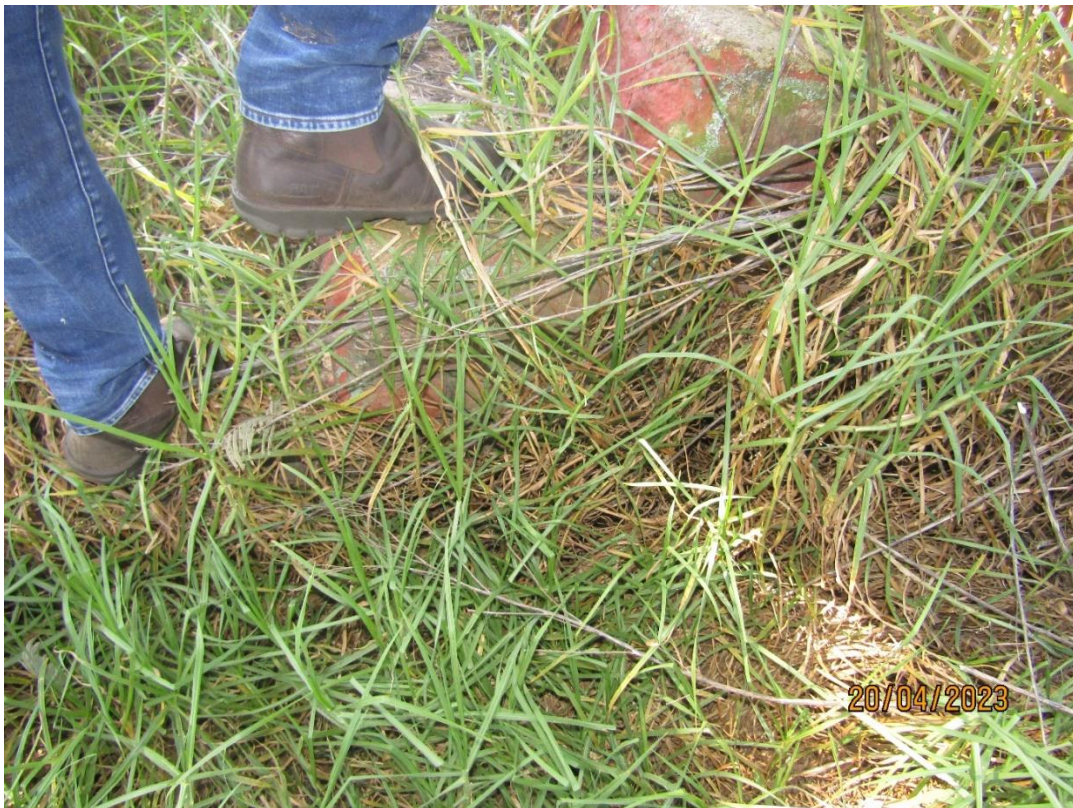
Figure 18: A closer inspection of the stone bricks that were used for the construction of the dilapidated old structure.
