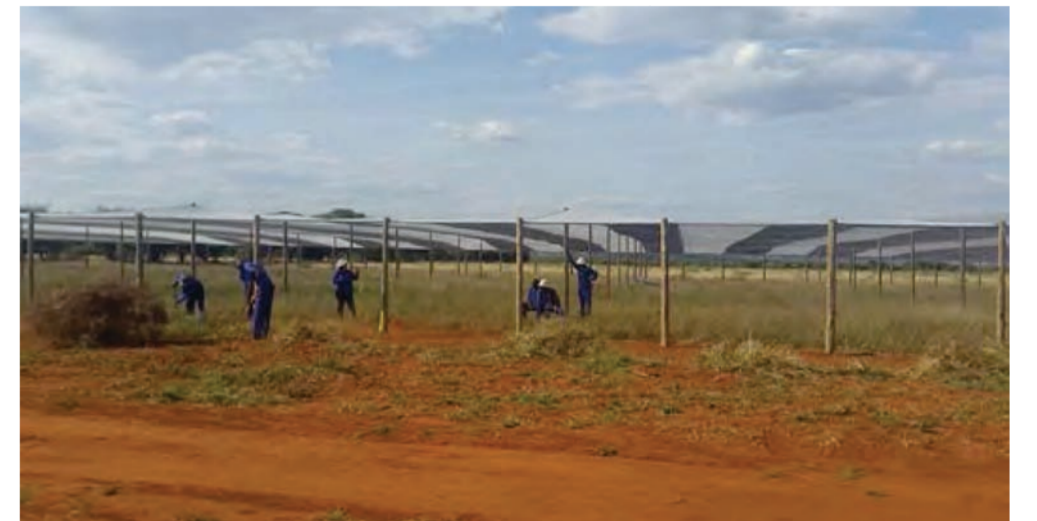
2nd Group of Beneficiaries removing weeds and clearing site in their Structure.
