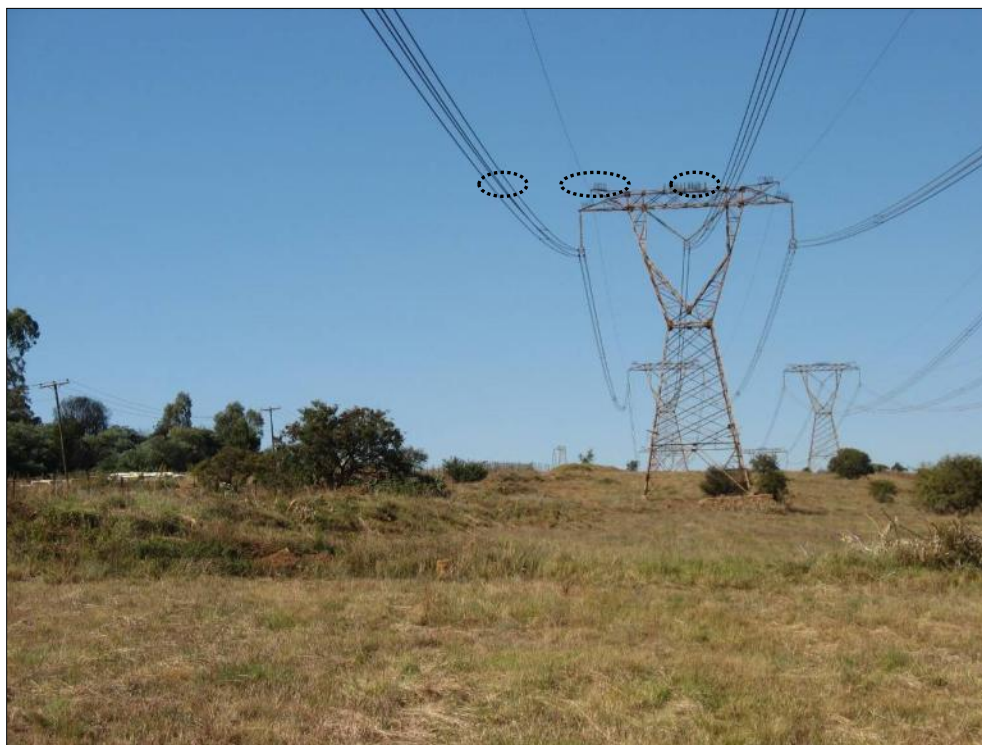
Figure 4-2: Bird guards (‘spikes’) fitted to a self-supporting tower.
