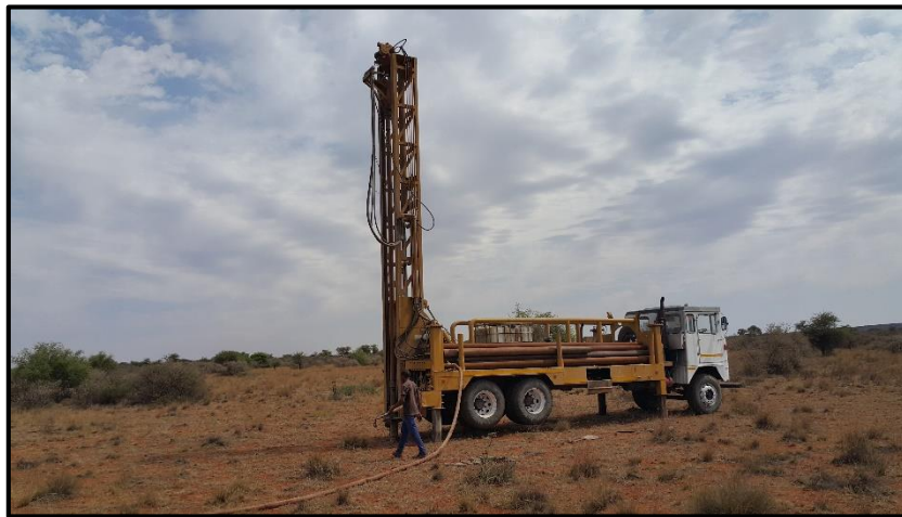
PHOTO 3: PERCUSSION DRILL RIG POSITIONED ON THE DRILLING POSITION, READY TO START DRILLING.
