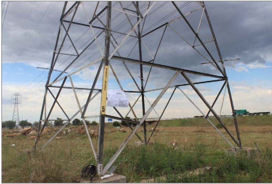
Figure 2a: Site notice attached to pylon of overhead powerline located in the centre of the site
