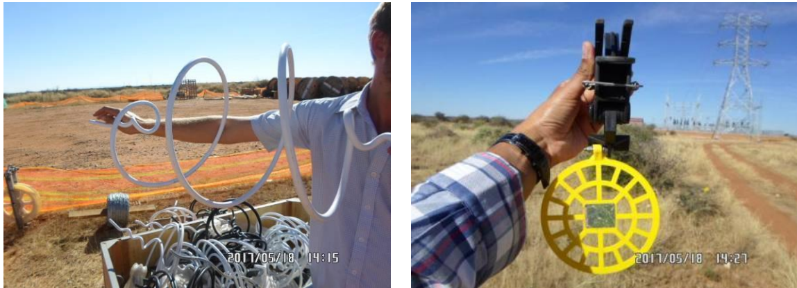
Figure 15: Examples of bird flight diverters to be used on the power lines: Double loop bird flight diverter (left) and Viper live bird flapper (right).
