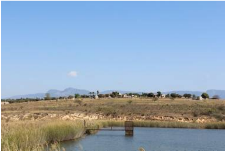
Photo 3: Dam embankment (upslope). The reeds will be removed from the upslope embankment and spillway as part of rehabilitation works.
