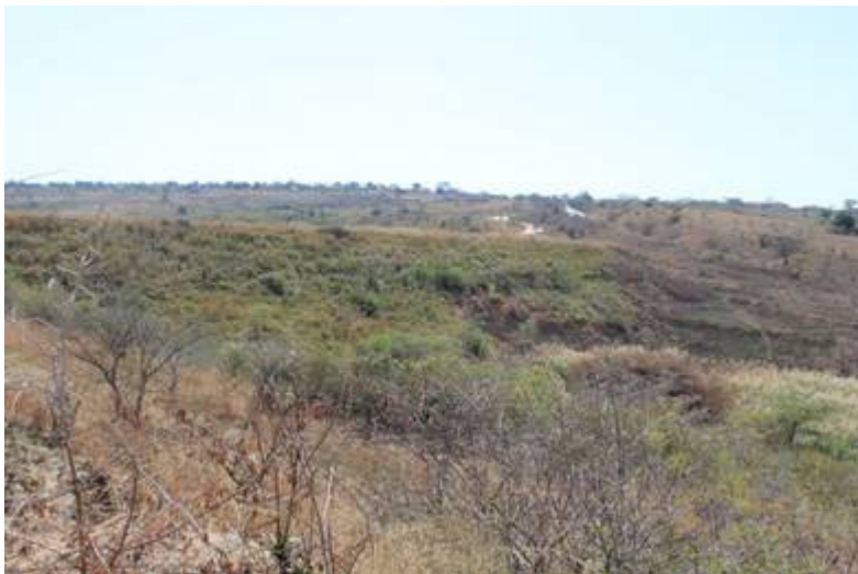
Photo 5: Downstream slope of dam embankment where rehabilitation works are proposed. Photo taken facing north towards the embankment.
