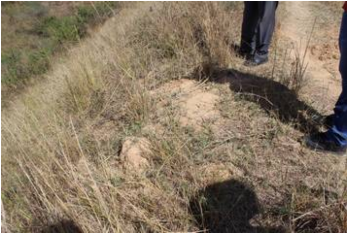
Photo 9: Termite nest on the dam downstream slope
