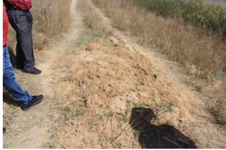
Photo 10: Termite nest on the dam crest
