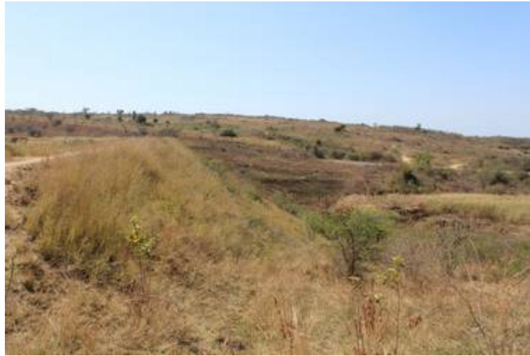
Photo 4: Downstream slope of dam embankment where rehabilitation works are proposed. The embankment is mainly covered in re-established grass.
