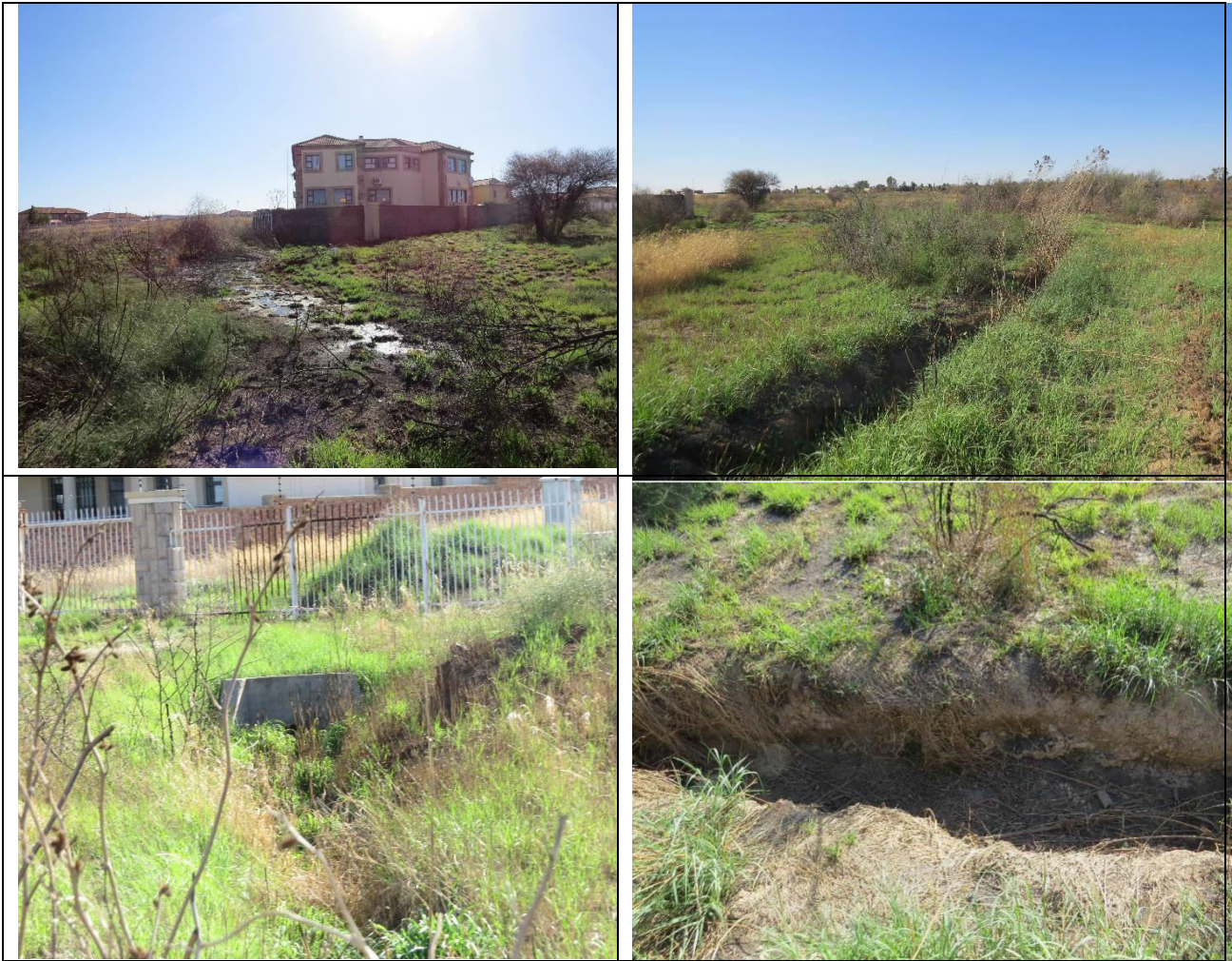
Figure 6: On-site investigation indicating increase in water inputs from the adjacent Fairview Estate and the surroundings from stormwater and sewerage leaks.
