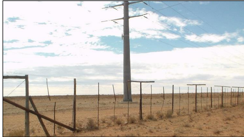
024 Single pole used for overhead lines
