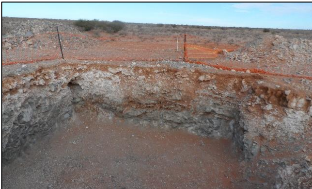
1 Foundation transmission pole
