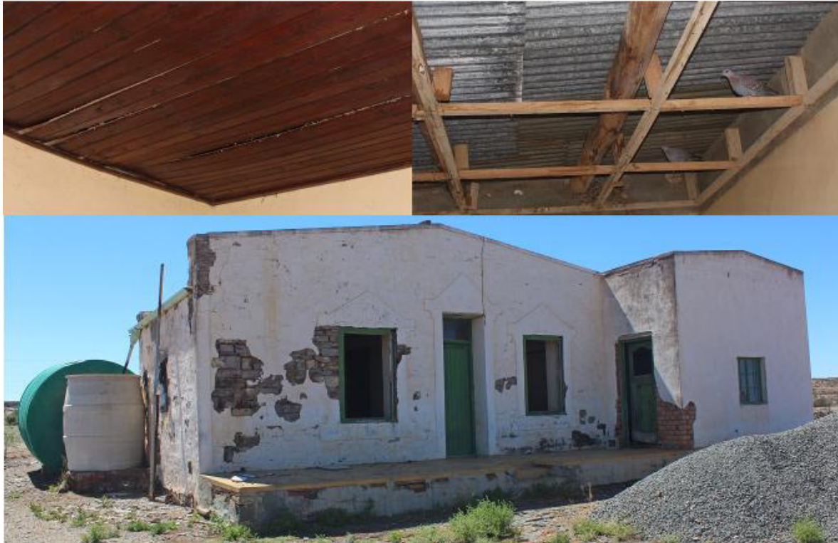
Figure 3-17: Photographs of the abandoned farmhouse and features relevant for potential bat roosts.
