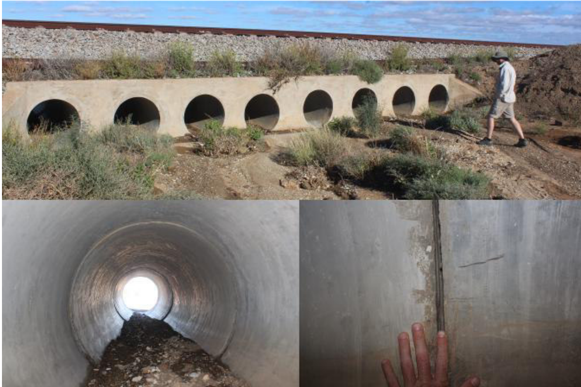
Figure 3-13: Photographs of the railway water underpasses and features relevant for potential bat roosts.
