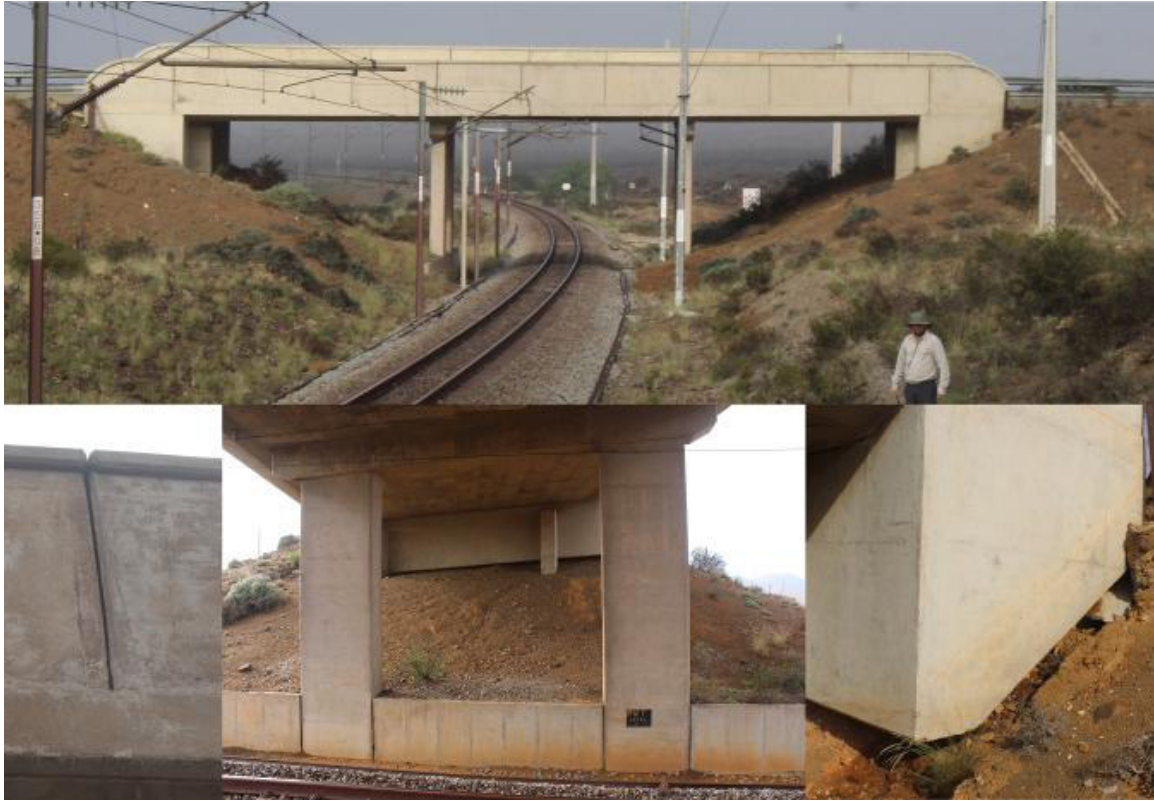
Figure 3-15: Photographs of the railway road overpasses and features relevant for potential bat roosts.
