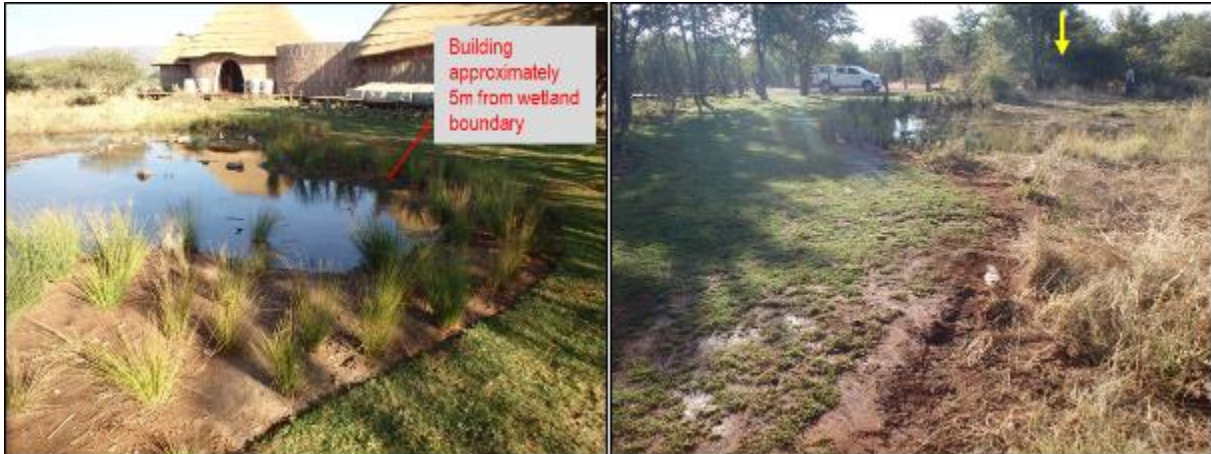
Figure 20: (Left) the delineated boundary of the wetland as per the SAS site visit in July 2019, is within 5m from the constructed building; (right) the locality of the eye of the spring indicated by the yellow arrow, from where the groundwater is piped.
