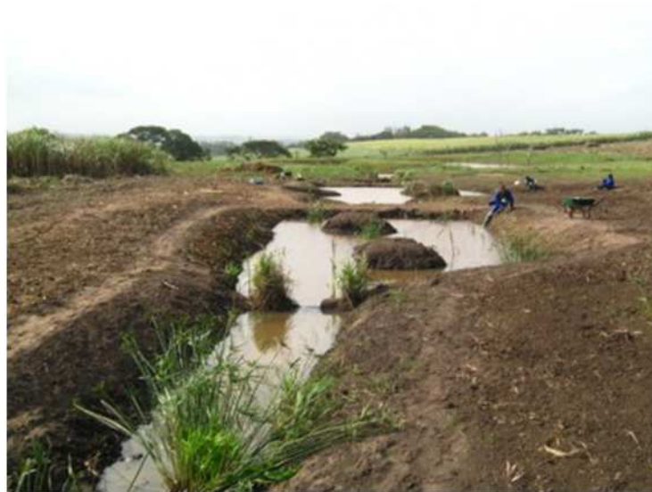
Example 2: Example of 'Soil Plugs' designed to deactivate small/shallow artificial drains at a wetland in the Ballito area (Source: Eco-Pulse).
