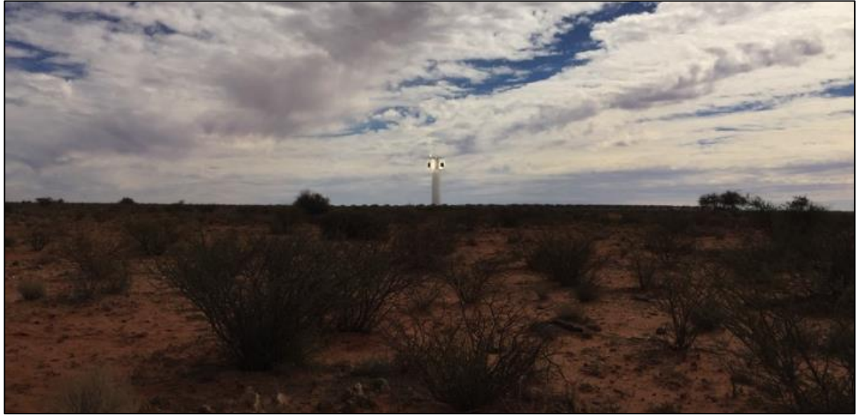
Figure 17: Survey Point 17 photograph taken to the north from the gravel road access to the under construction Sirius Solar PV Project One facility.
