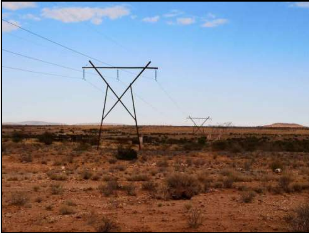
Photograph 1.3: Oasis-Orange Eskom 132 kV line
