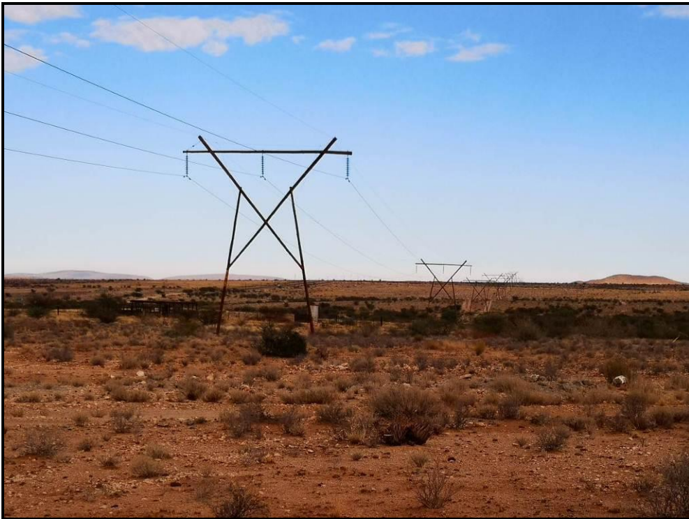
Photograph 1.3: Oasis-Oranje Eskom 132 kV line
