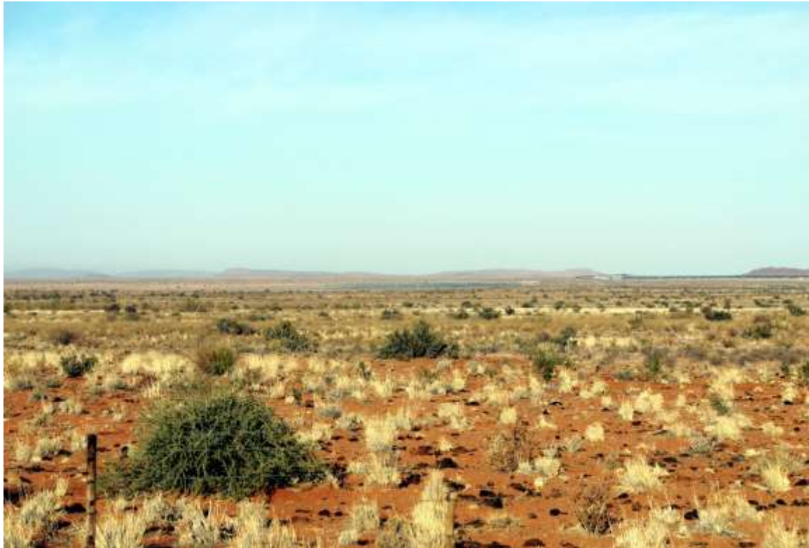
Plate 6, View of Sirius Solar PV project under construction (centre picture) from the Lutzputs Road.
