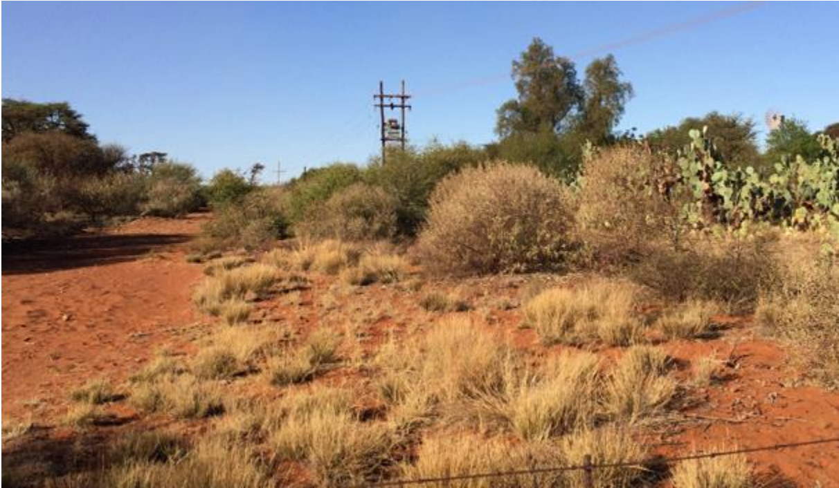
Figure 26: View north from Photo 7 location of the existing distribution line which the proposed 132kV power line will cross over.
