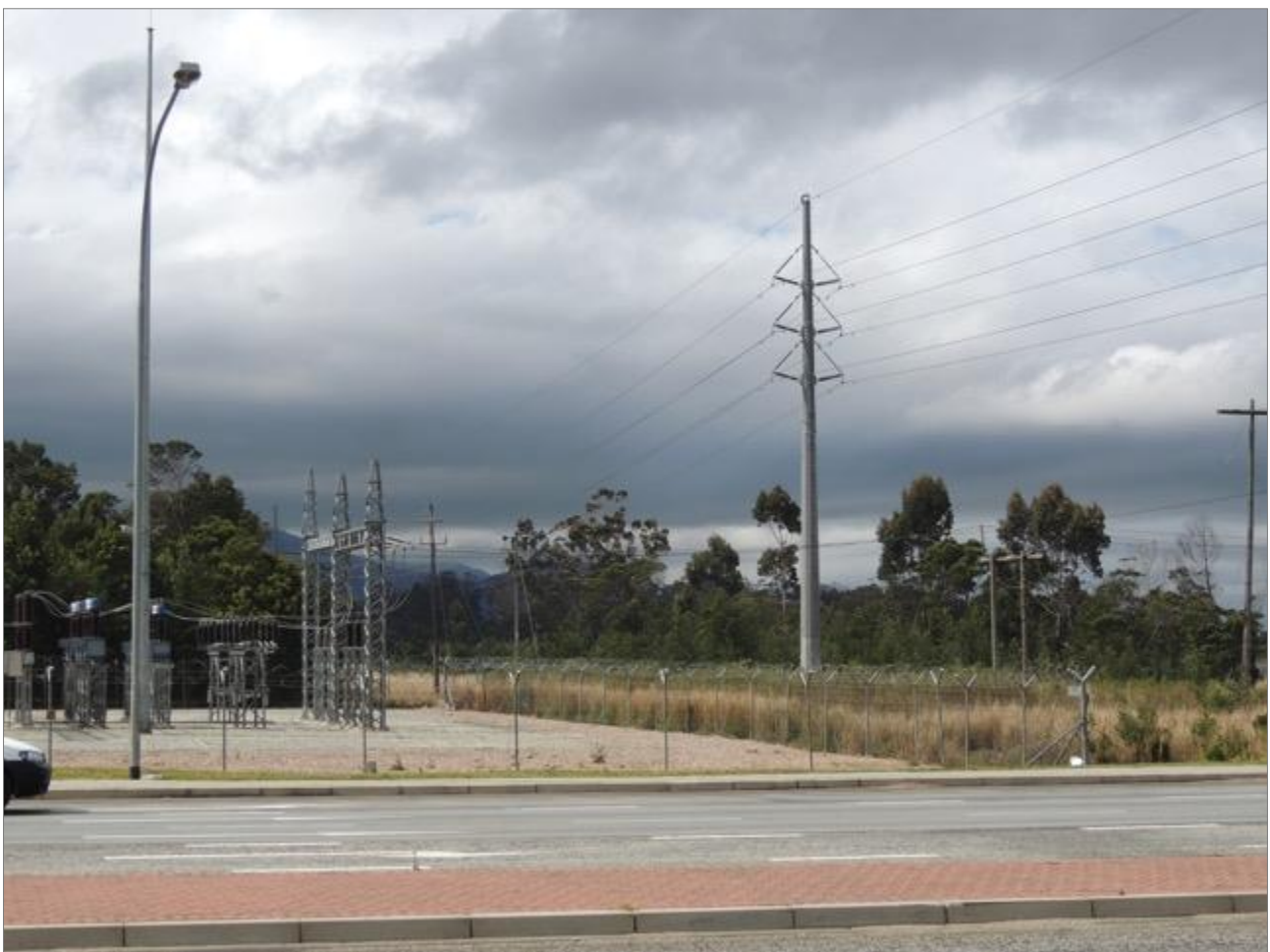
Figure 5: Example of transmission lines link to a small substation (Source: VRMA)
