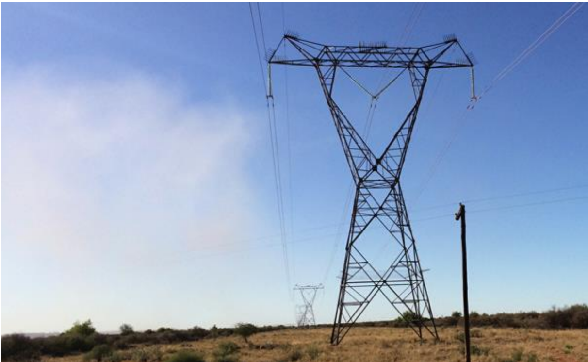
Figure 25: View northwest from Photo 6 location of the existing Eskom power line under which the proposed 132kV power line will be routed.
