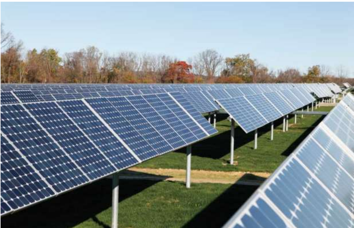
Figure 3: Photographic example of a similar PV technology (Solar Professional)
