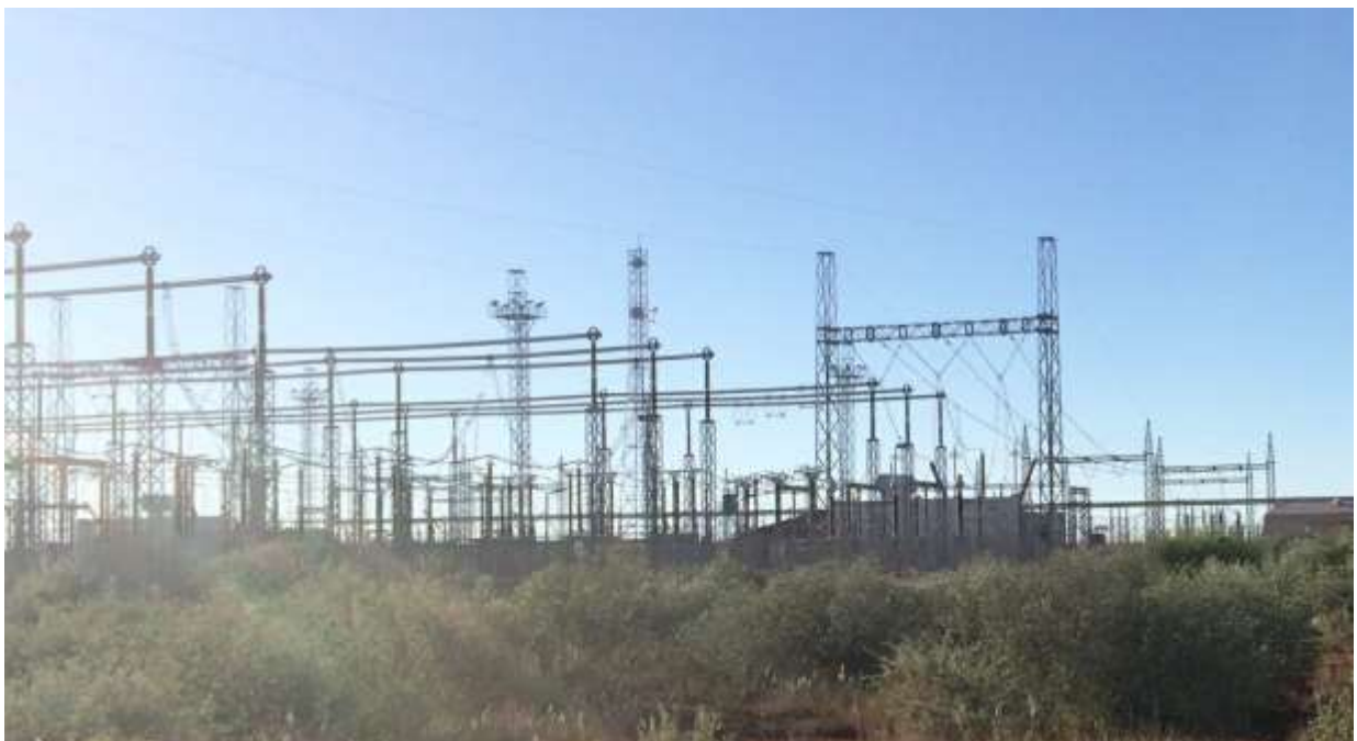
Figure 15: Photograph of the existing Eskom Mookodi Substation
