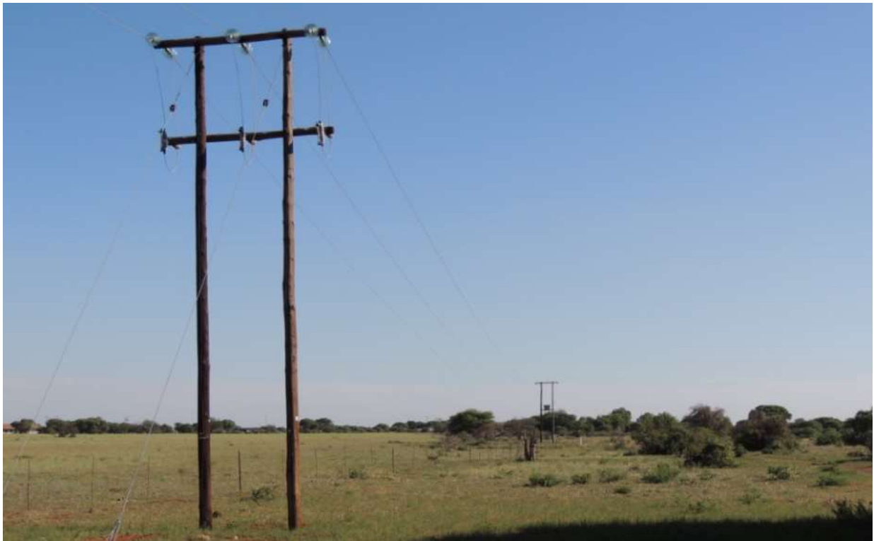
Figure 14: Photograph of the existing Eskom line along which the proposed power line is to be routed.
