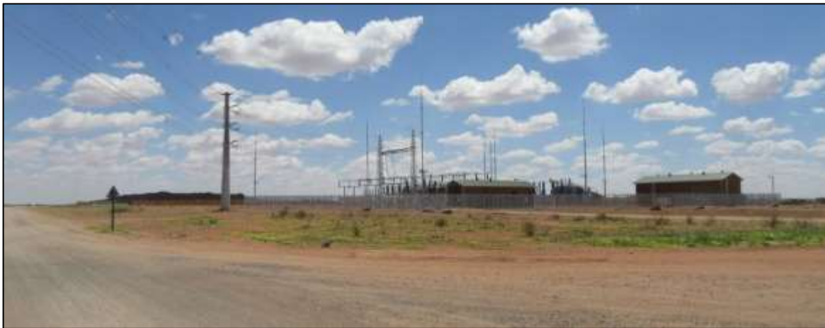
Photograph 3.12: Substation and 132 kV line on Dayson’s Klip farm located just to the west of Scatec’s newly commissioned Daysonsklip 1 SEF
