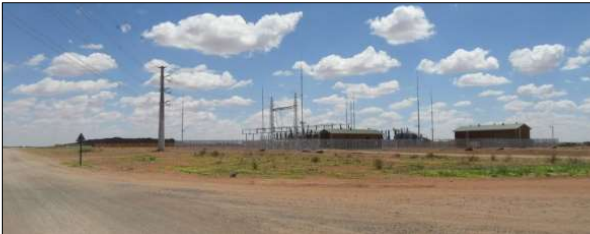
Photograph 3.12: Substation and 132 kV line on Dayson's Klip farm located just to the west of Scatec's newly commissioned Daysonsklip 1 SEF
