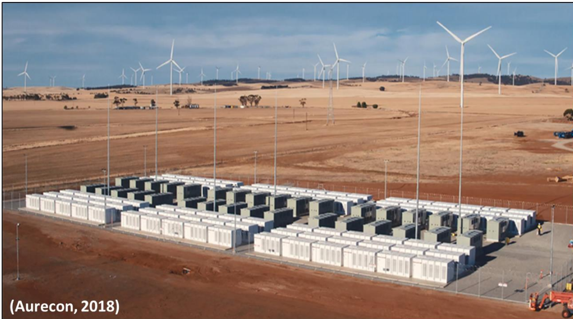
Figure 2: The 100 MW/129 MWh Li-ion battery coupled with the Hornsdale wind farm in Australia.
