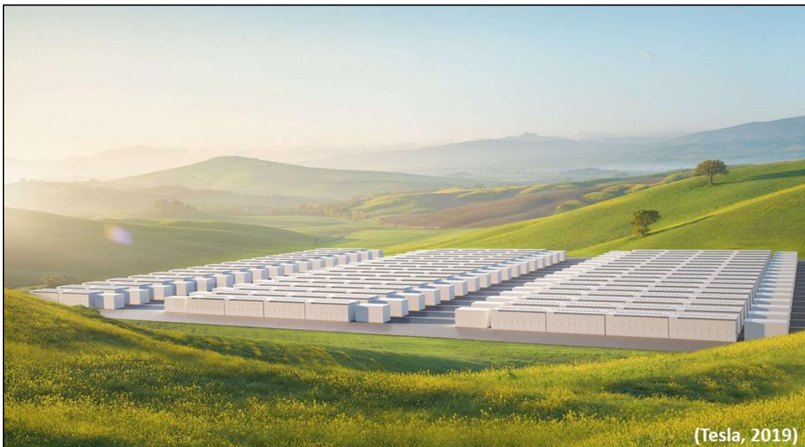
Figure 1: Tesla's Megapack Li-ion Battery (Modular System).
