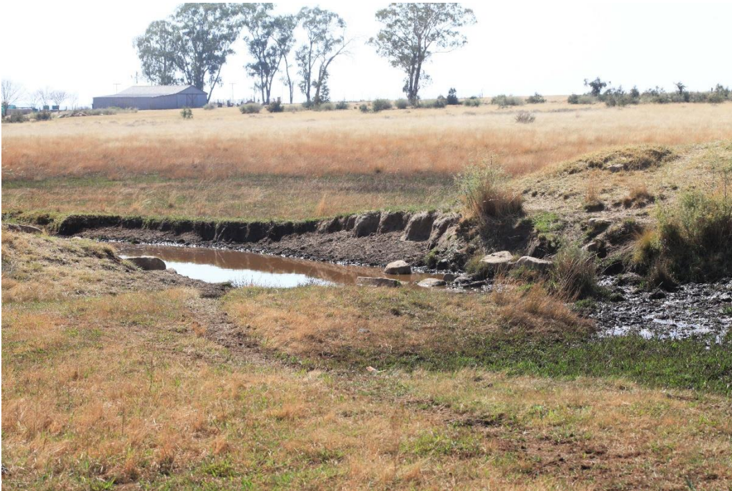
Photo 6 Broken groundwater of small in-channel dam at the site. Photo: R.F. Terblanche
