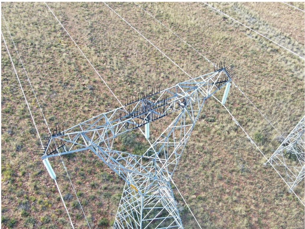
Figure 4: High voltage powerlines running through the Project Site.
