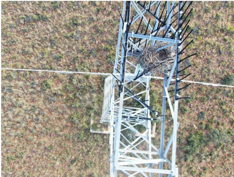
Figure 8: Jackal Buzzard nest on high voltage powerline pylon in the Study Area.
