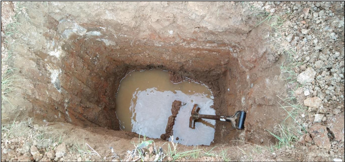
Photograph 8: Water Seepage and Material Encountered in TP205
