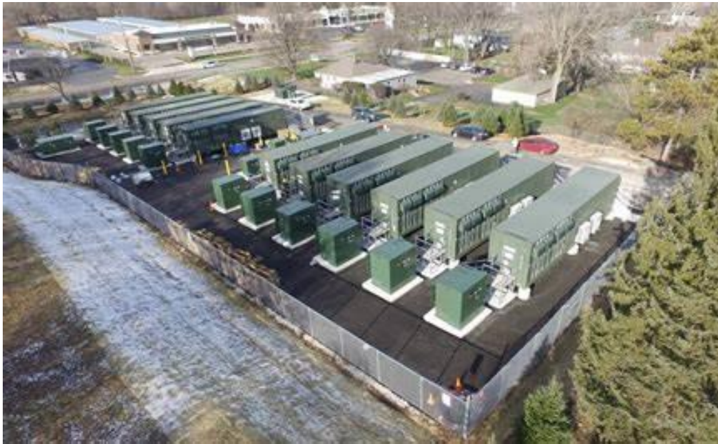
Plate 1 - Typical Battery Energy Storage System
