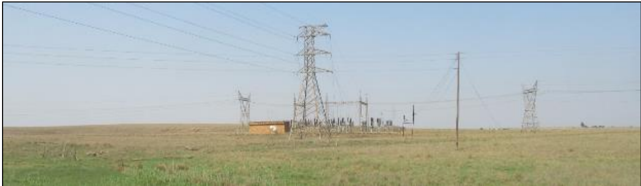
Photograph 3.4: Substation located on Bosjesspruit 291/RE to the west of the Trichardt-Charl Cilliers Road 6 km east of the site
