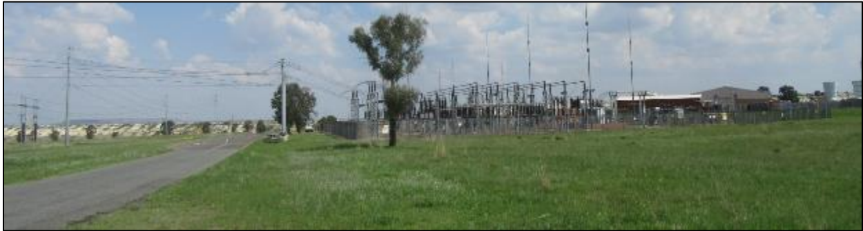
Photograph 3.18: 132 kV lines entering Zandfontein substation
